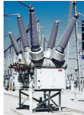
circuit breaker (can break short-circuit current)
