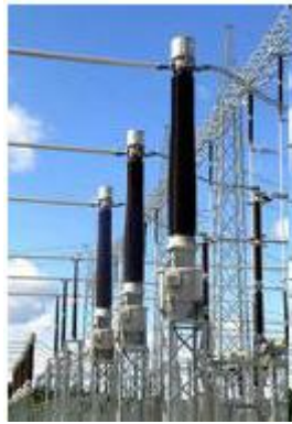
current measurement transformers
