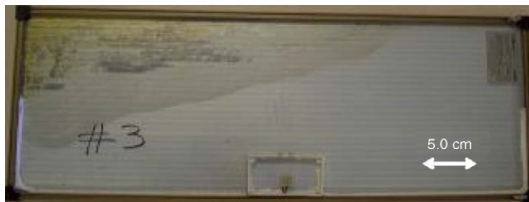
Fig. 3. Photograph of rear of module showing delamination and moisture ingress.
